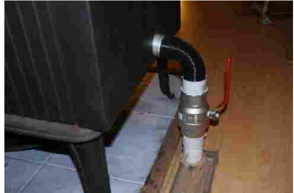
Fig 2. Flexible aluminum duct and ball valve at the back of the stove. Aluminum duct is cold to touch when the wood stove is hot.
