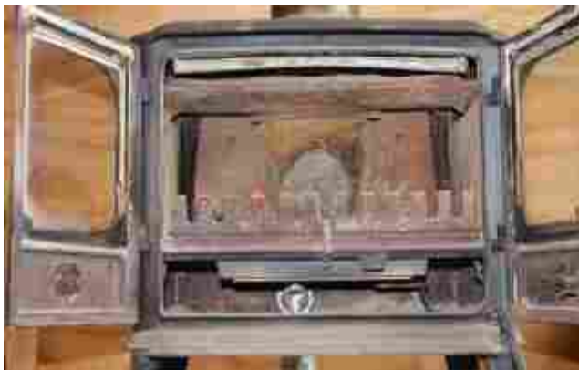
Fig 1. Cold air intake at the back of the ash compartment underneath the firebox (ash tray removed) after a few months of use. Note a shiny appearance of the duct with no trace of smoke presence. The stove is 10 years old.
