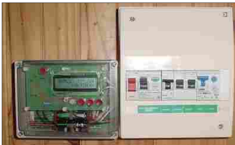
Tom's energy meter (modified Altronics kit) installed indoors next to the switch box, enables him to monitor power and energy use
